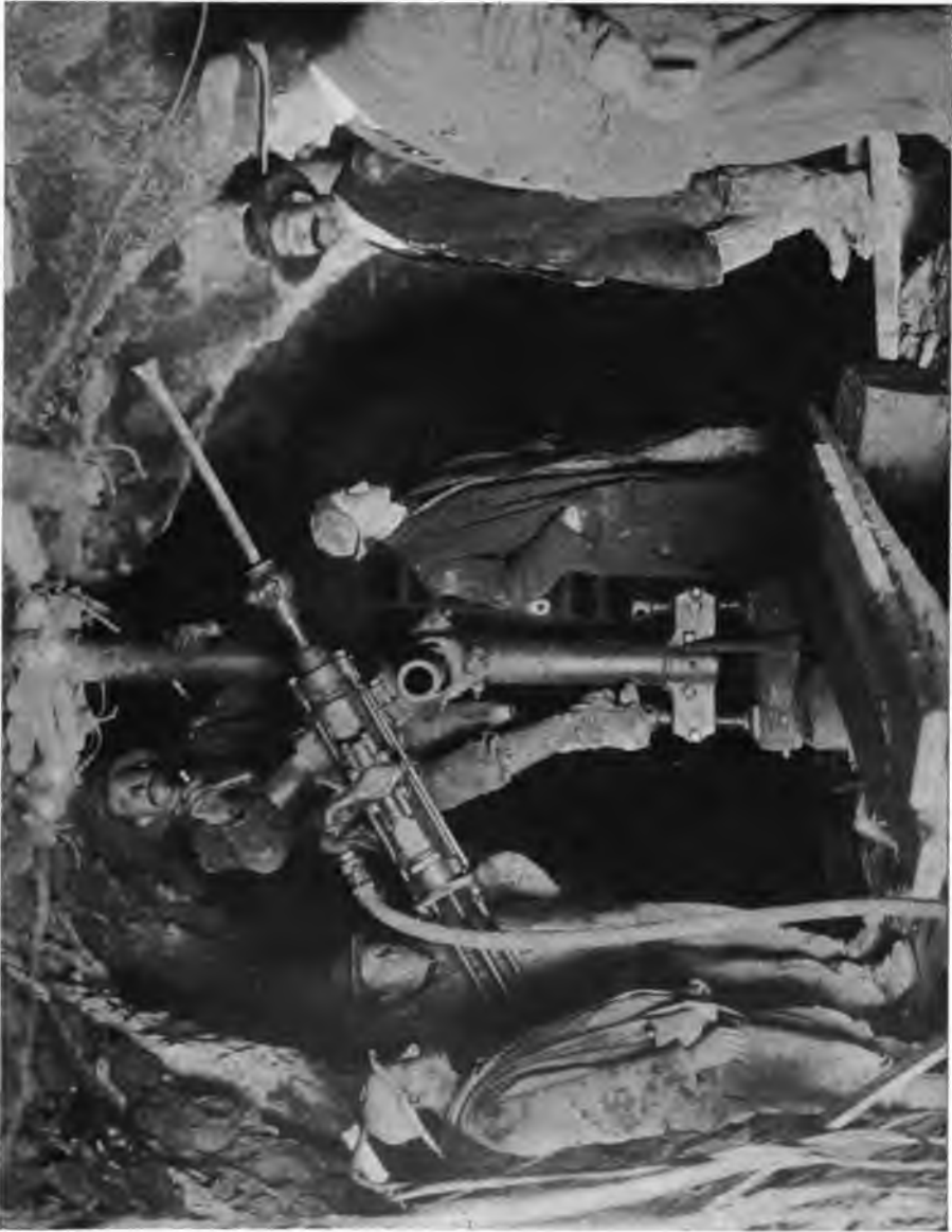
PLATE 120.—Contract 47. Compressed-air Drill as Mounted on Column and Arm in Heading of Wallkill Tunnel. Usually headings were drilled by four drills mounted on two columns.
